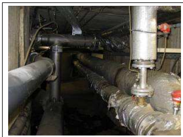
Figure 3 – The insulated pipework running from bottom right to the centre of the image is the longitudinal continuous flow pasteurisation plant
