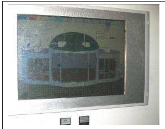
Figure 12 – One of the visual interfaces of the central control and monitoring software. Touch screen control allows various operational parameters to be changed and monitored
