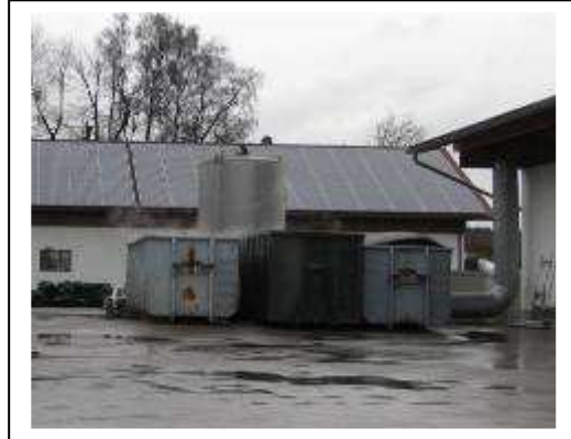
Fig 14 – The large metal duct on the right of the image directs heat to the covered containers for the drying of wood
