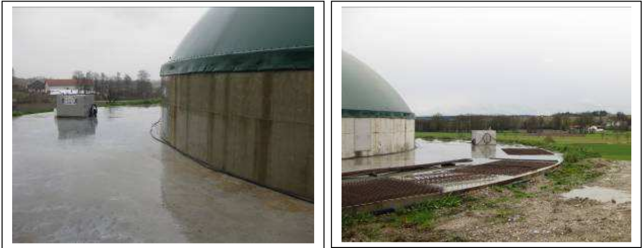
Figure 8 & 9 – Top of primary digester (Outer ring) with mixer service box. Above ground section of digestate & gas storage (Inner ring) also visible.
