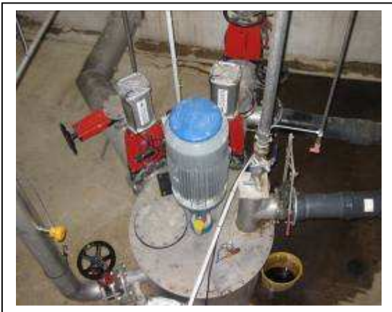
Figure 11 – Central pumping station which controls the flow of substrate between digesters and stores
