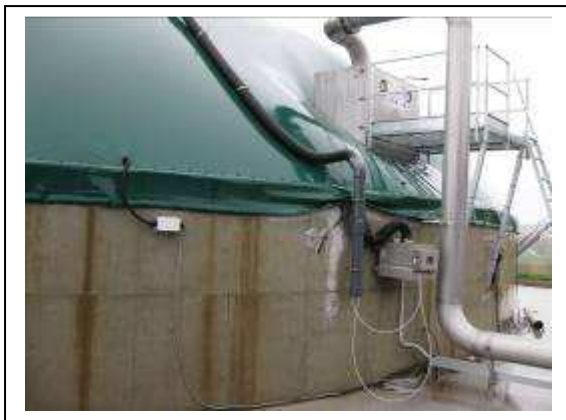
Fig 15 – The above ground section of the “Inner Ring” digestate store with quarter dome gas storage above. The stainless steel box is the service box for the internal hydraulic mixer, and the stainless steel
