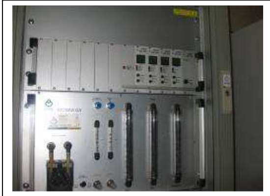
Fig 13 – Stationary gas analyser monitoring the quality of gas produced by the digestion process prior to combustion within the CHP units
