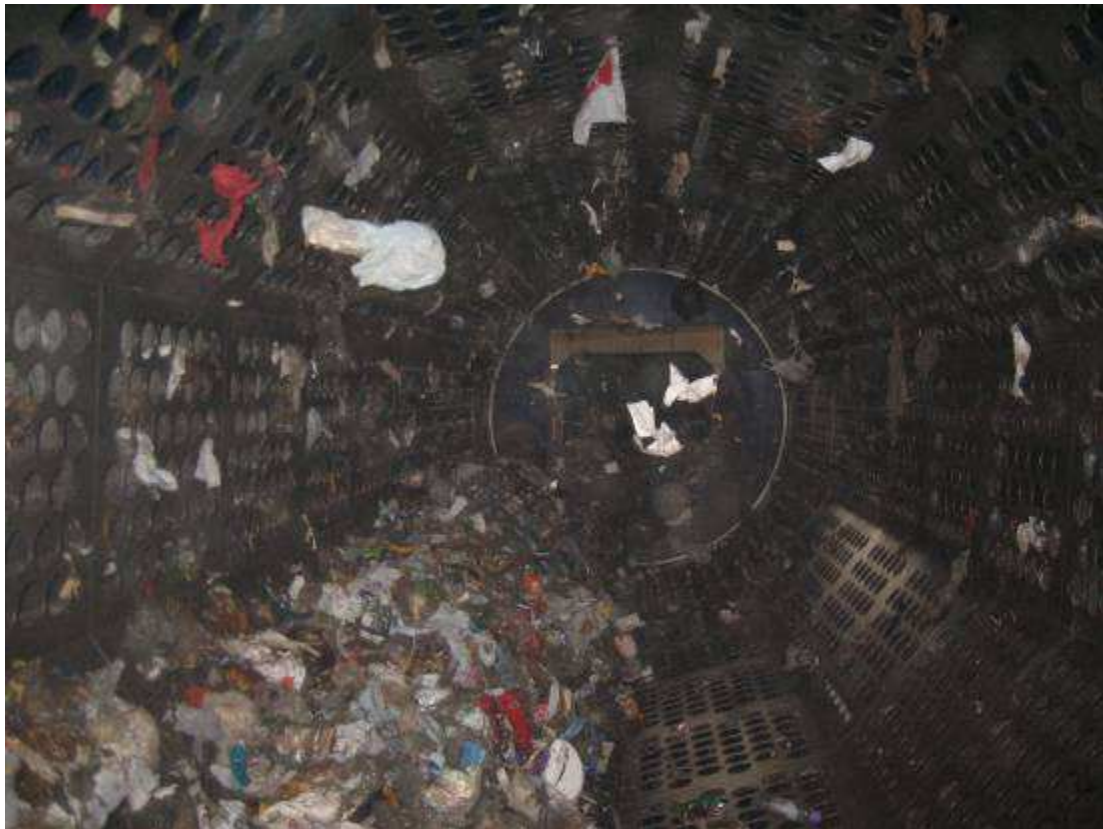
Figure 7 Inside trommel sieve at Heilbronn
