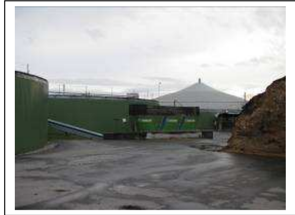
Figure 18 – General site layout showing one of two primary digesters to the far left, secondary fermenter and solids feeder in the centre and digestate storage to the right.
