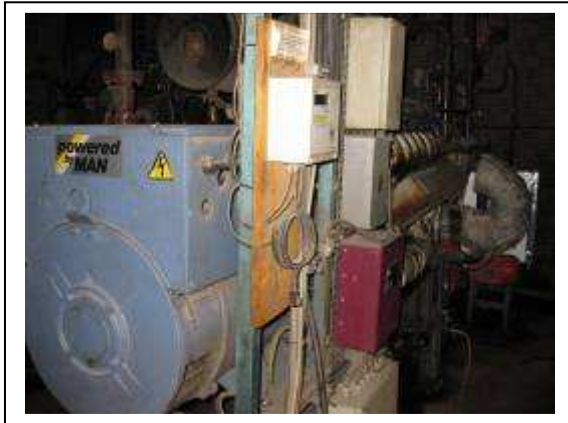
Figure 10 – One of three CHP engines
