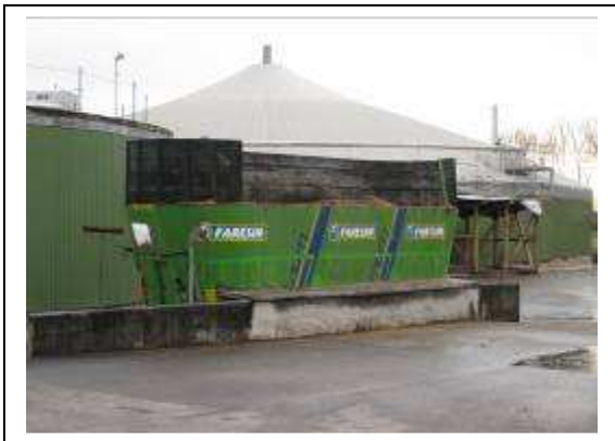
Figure 15 – Solids feeder unit with digestate storage tank visible to rear
