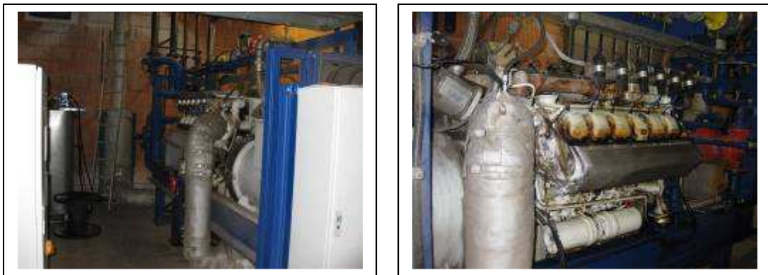
Figures 22 and 23 – CHP engines used at the energy crop plant
