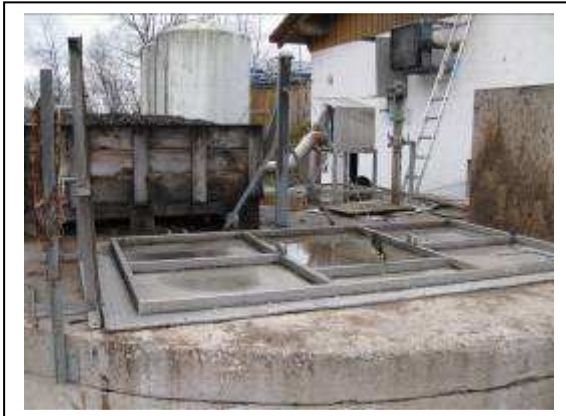
Figure 1 – Below ground concrete reception tank for non ABP substrates
