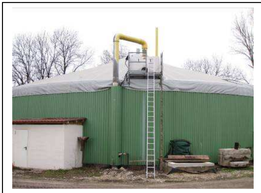
Figure 11 – First digestate storage tank with flexible membrane roof, yellow gas collection pipe and service box for mechanical mixer
