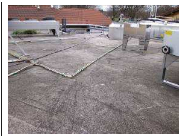
Figure 6 – Concrete roof of digester No. 1 with hydraulic lines to mixers and heat exchangers for dissipating excess heat
