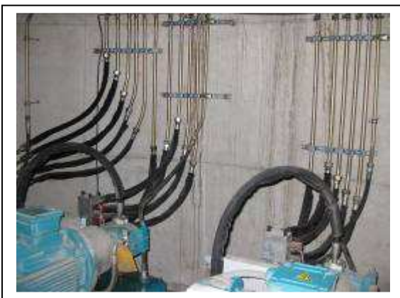
Figure 20 – Hydraulic compressors located in central control room with hydraulic lines which link to hydraulic mixing motors in digesters.
