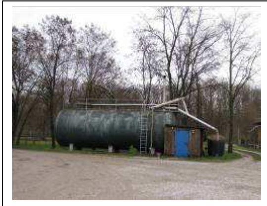
Figure 2 – Above ground cylindrical tank for substrates containing ABP material
