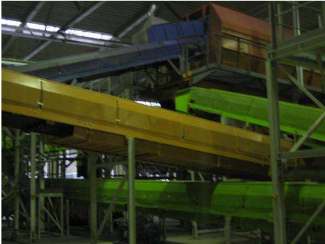
Figure 6 Conveyors between mechanical separation stages
