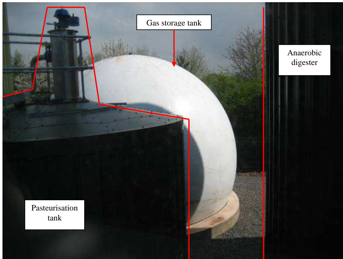
Figure 7 Pasteurisation tank (with gas storage tank in background and digester on the right)
