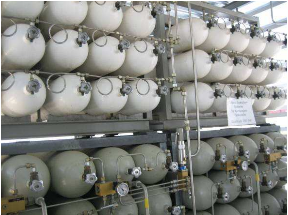
Figure 9 Biogas storage at filling station at Otelfingen
