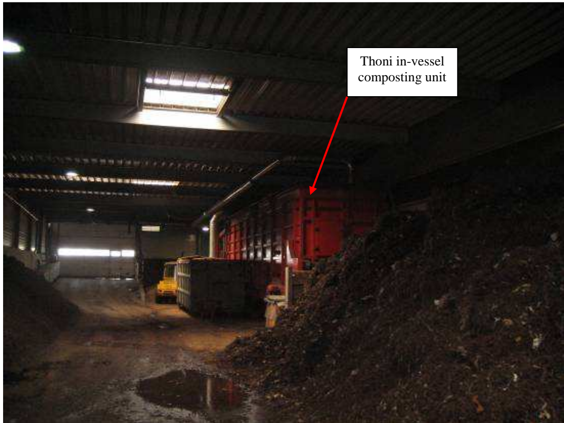
Figure 6 Thoni in-vessel composting system at Otelfingen
