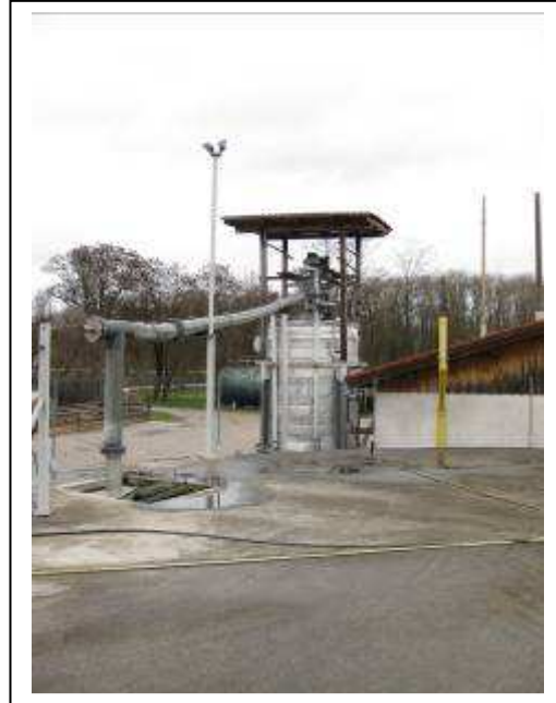
Figure 4 – Pasteurisation unit looking to the south west showing gas connection pipe to digester No.3
