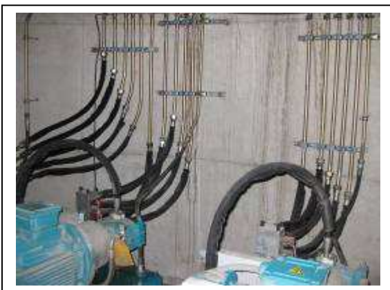
Figure 20 – Hydraulic compressors located in central control room with hydraulic lines which link to hydraulic mixing motors in digesters.
