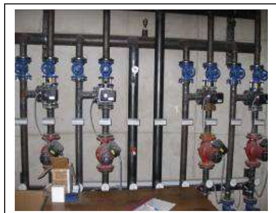
Figure 21 – Heating manifold located in central control room which distributes heated water to digesters.
