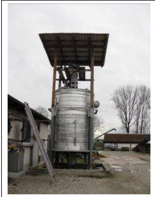
Figure 3 – Pasteurisation unit looking northwards
