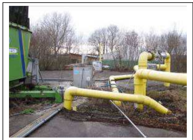
Figure 7 – Concrete roof of digester No. 2 with yellow gas collection pipes and stainless steel service boxes for hydraulic mixers
